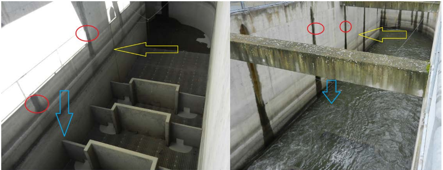
Figure 3: Lower three weirs at the JD-S fish ladder during winter maintenance (dewatered) on left, and during operation (watered up) on right. Yellow arrows show the same seam in the fishway wall, red circles indicate same water stains. The blue arrows show the location of the third weir proposed for removal. The high water line (not the same as the current water depth), along the wall, can also be used as an indicator.
